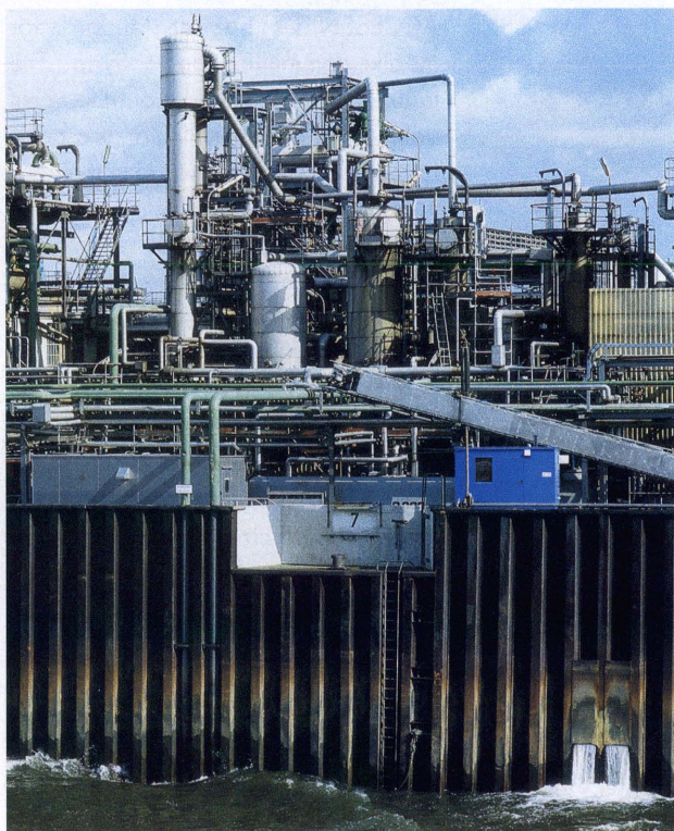
FIG 1 Automatic water analysis system from Rohde & Schwarz Cologne accommodated in an easily transportable, bright blue container to be set up on site
